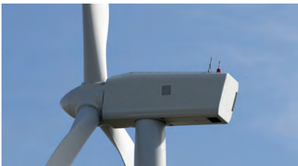
Figure 38 : Wind turbine nacelle
